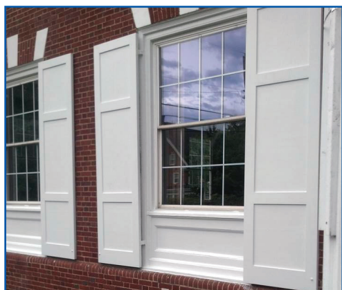
Repainting the chapter house's exterior was one of the projects completed during the summer.
